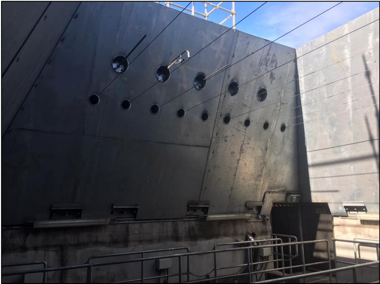
Figure 1: Inside URVF Vent 1
