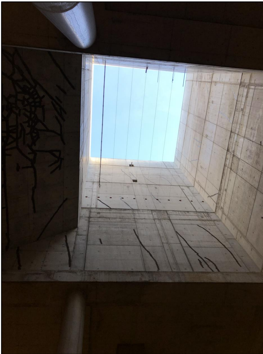
Figure 3: Inside PRVF Vent A
